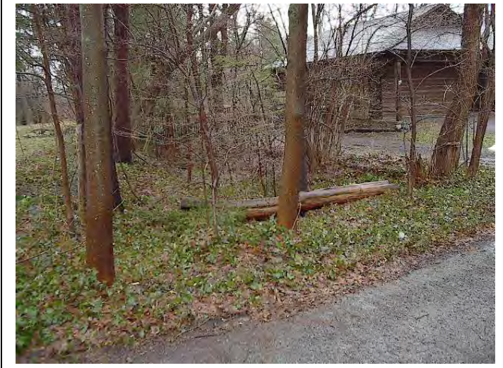
Non-functioning emergency spillway for Carpenter's Pond.
